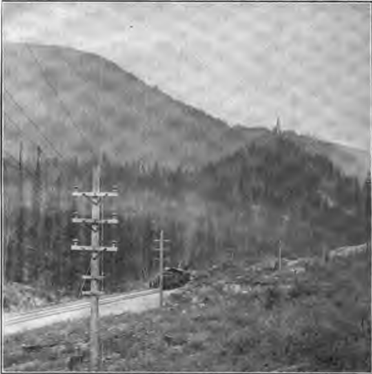
FIG. 7.—General view of transmission line
